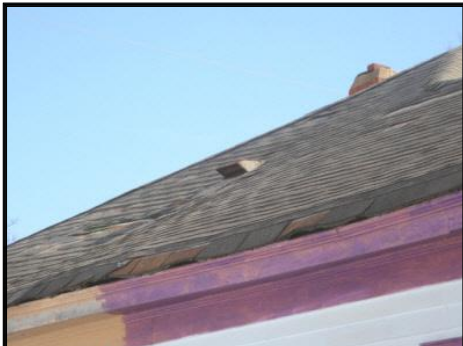
roof-wavy, damaged/missing shingles
