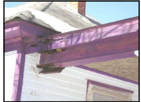
damaged porch roof
