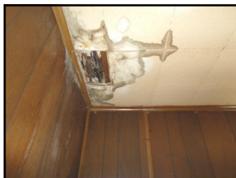
water damaged ceiling
