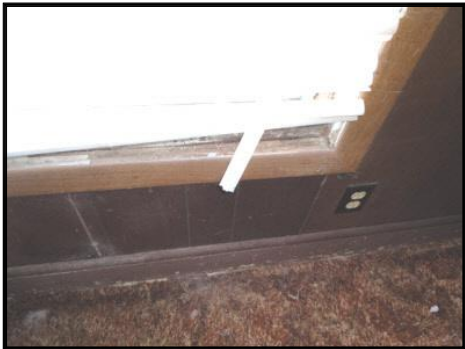
Rotted interior window sills
