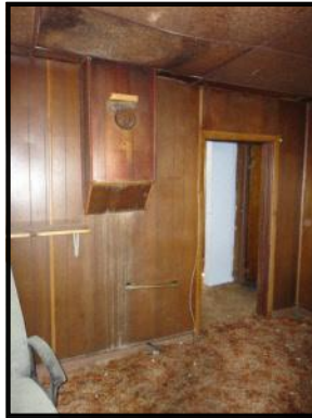
missing gas heater
