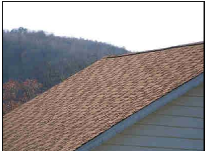
Roof is nearing the end of its useful life.
