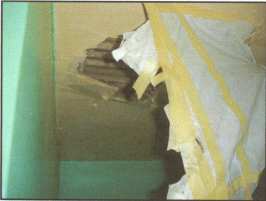
Hole in Bedroom Ceiling
