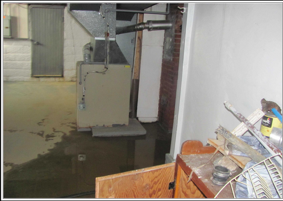
Basement (Water penetration)
